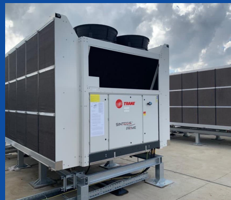
Equinix Datacenter - United Kingdom
